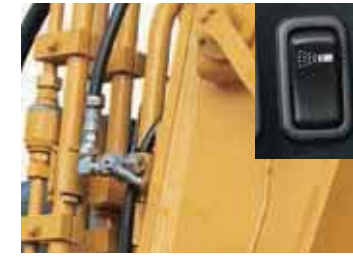
Dust suppression system (with drainage circuit) A drainage circuit is installed to drain water from the lines and prevent rust or freezing.
